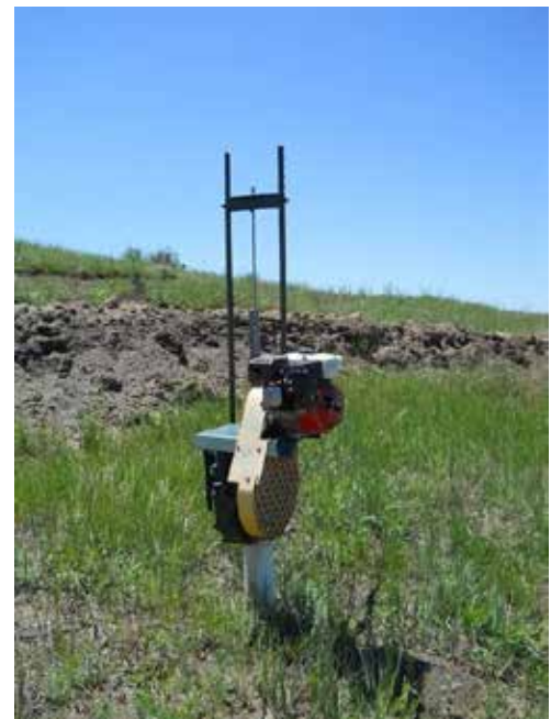
Groundwater monitoring well at Crow Butte Resources Inc., Dawes County.
