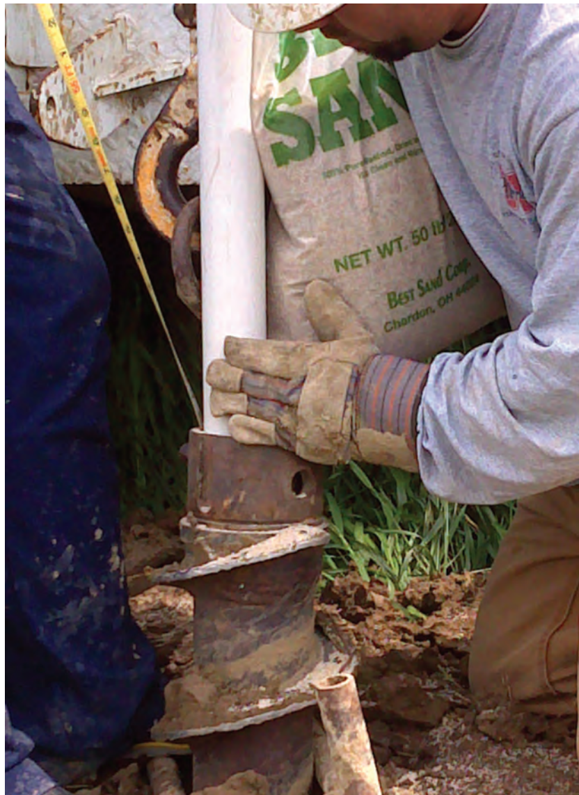
University of Nebraska Conservation and Survey Division staff installing a monitoring well near Clearwater, NE.
