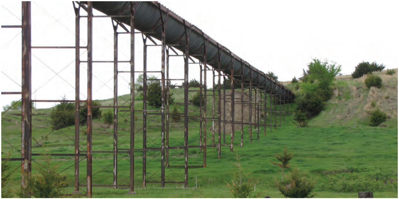
Taylor-Ord canal, property of North Loup Public Power and Irrigation District, located north of Elyria, NE.
