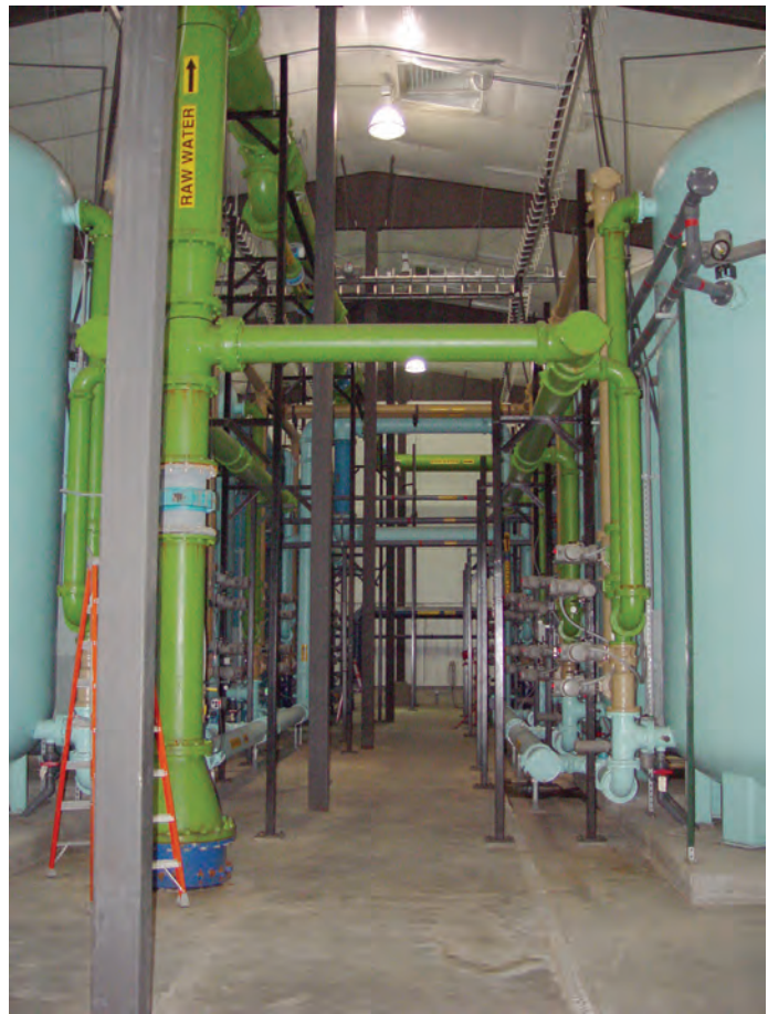
Ion Exchange plant to remove uranium (McCook, NE).
