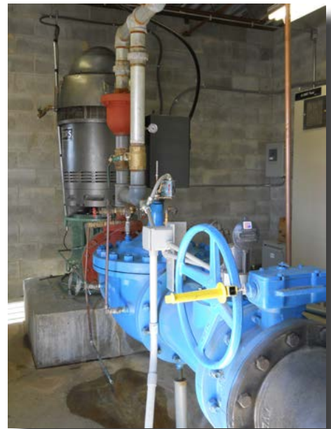
Public Water Supply well capable of pumping thousands of gallons per minute (Hastings, NE).
