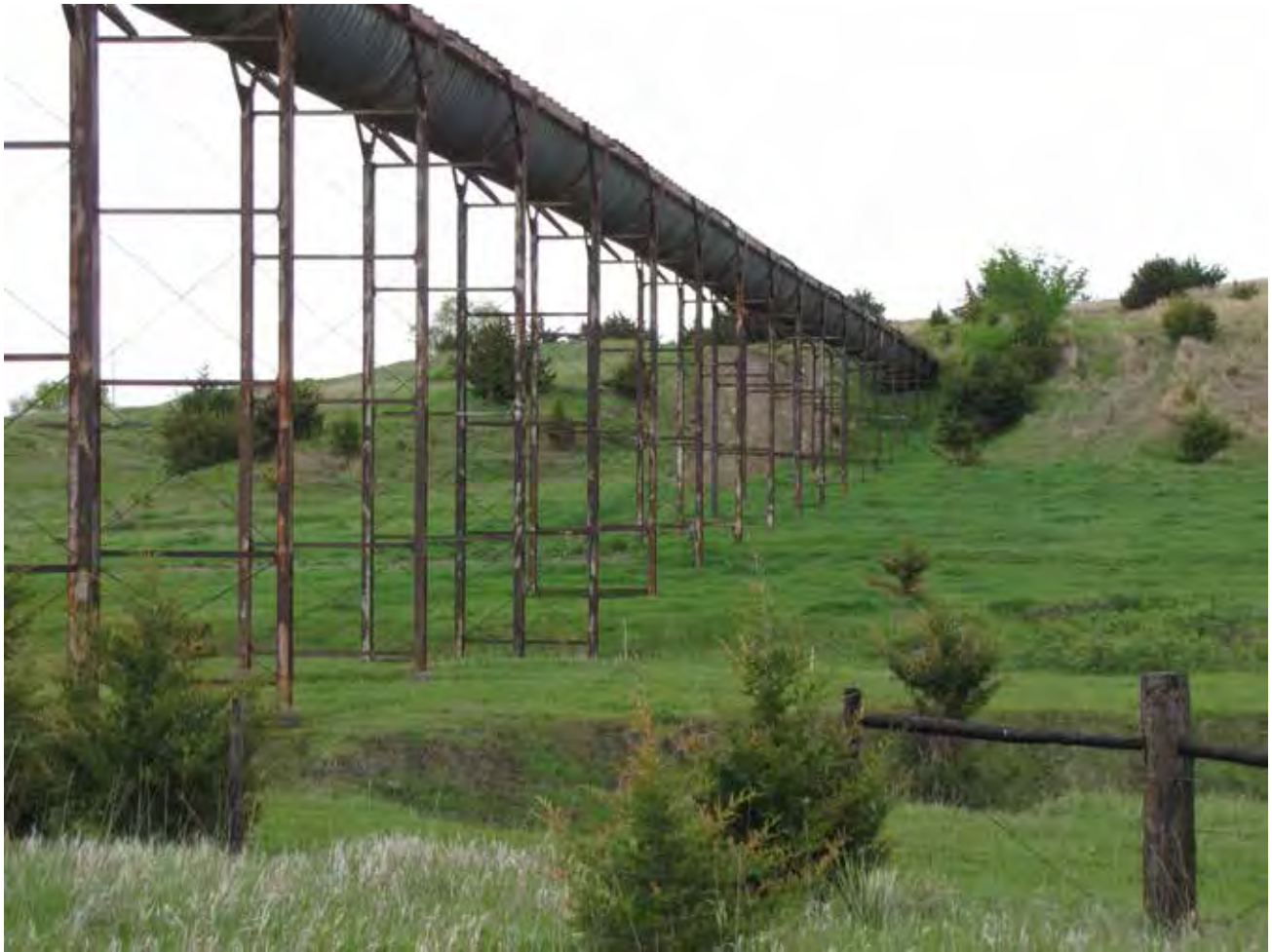
Taylor-Ord canal, property of North Loup Public Power and Irrigation District, located northwest of Elyria, NE.
