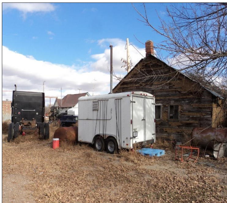
Air sparge/soil vapor extraction remediation system at the site of a former gas station.
