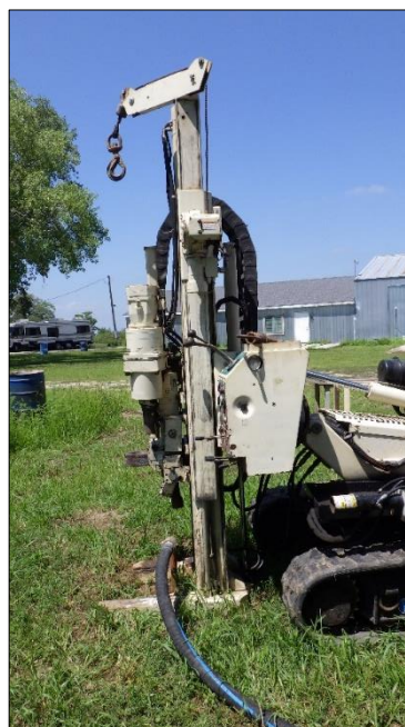
Photo shows a direct-push rig preparing for in-situ enhanced bioremediation injections into the aquifers beneath the Former Lincoln Air Force Base Atlas "F" Missile Site 1 in Elmwood, NE.
