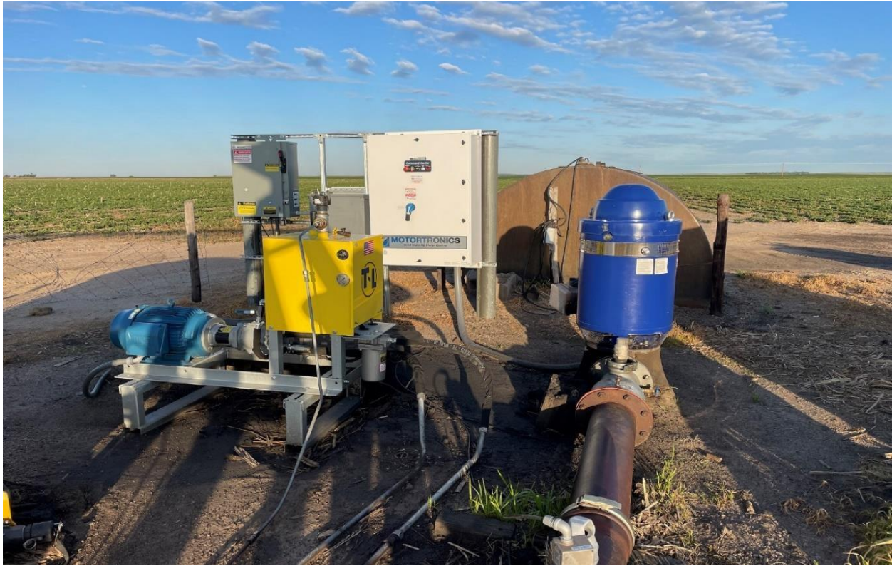
New electric motor and related equipment replacing a diesel engine at an irrigation well in Lincoln County, partially funded by the 2022 Nebraska Clean Diesel Rebate Program. Photo courtesy of the owner.
