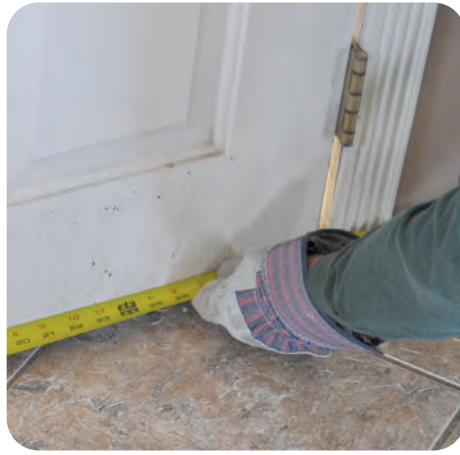
2. Measure door top or bottom as well for weatherstripping and potential door bottom or sweep
