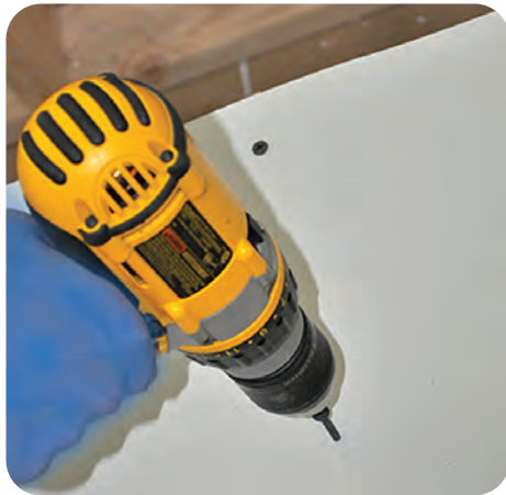
A-5. When support bracing has been used, screw infill material to bracing as well
