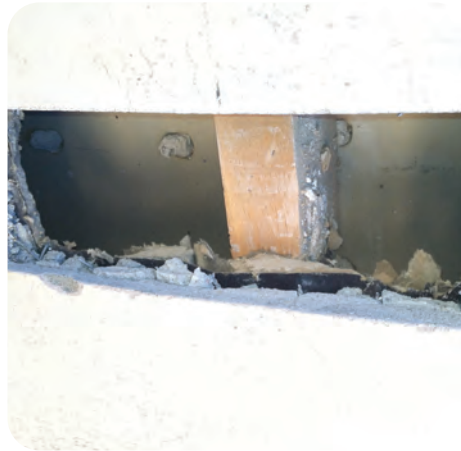
5. Drill holes as required based on building frame design and exterior materials
