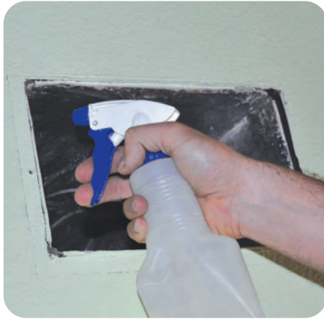
D-2. Clean the area around the duct boot to allow for better adhesion of fiberglass mesh tape
