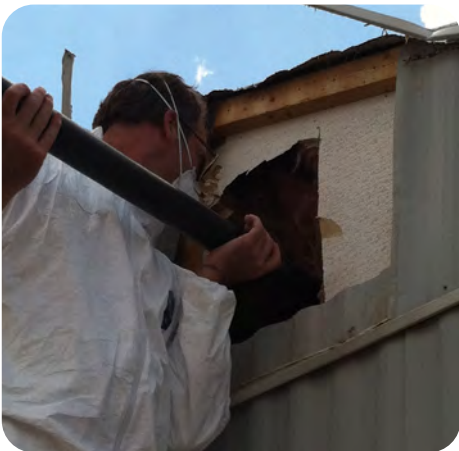
4. Insert blower hose as far as possible and then retract slowly to fill cavity entirely, on each side of marriage wall
