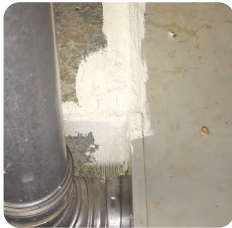
B-5. Apply additional mastic over mesh and tape, extending at least 1 inch past edges of tape in all directions
