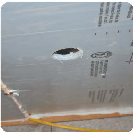
4. Cut an access hole into each cavity of the floor, large enough for fill tube
