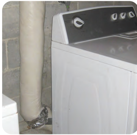
6. Duct in uninsulated space is insulated
