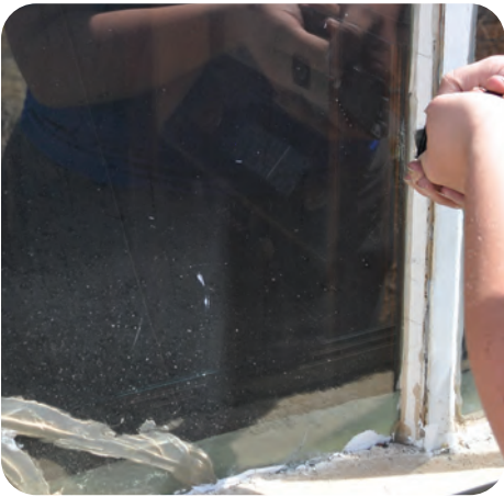
1. Remove all broken glass
