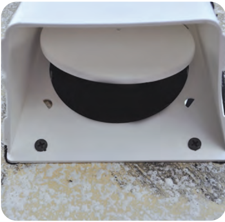
5. Termination has backdraft damper and no cage
