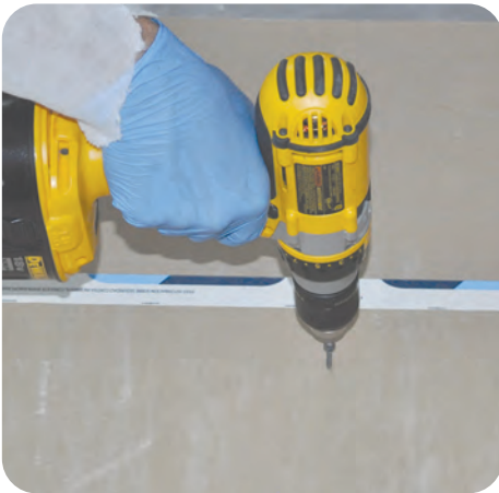
A-4. Place Infill material over opening and secure in place with mechanical fasteners
