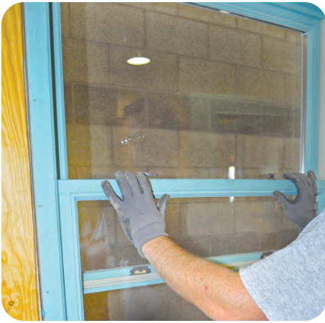
7. Ensure window is operational
