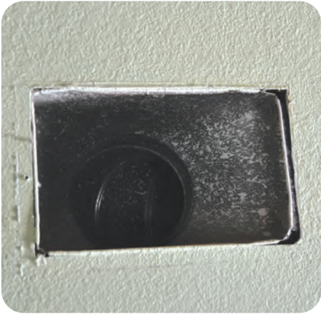
D-1. Often, holes for duct boots are cut too large and leave gaps around the boot as a path for air leakage
