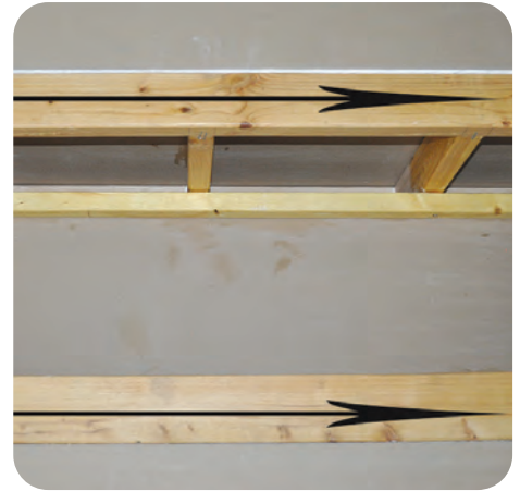
A-3. Apply sealant along top plates, bracing, and framing members adjacent to opening more than 24 inches apart
