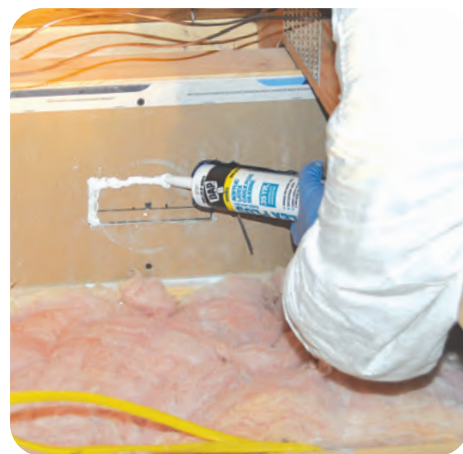
6. Seal access holes permanently and completely
