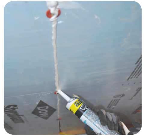
3. Seal seams between sheets of rigid material to prevent air movement and insulation leakage
