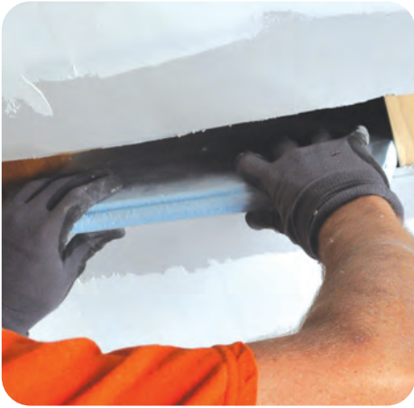
5. Blocking still needs to be put into place
