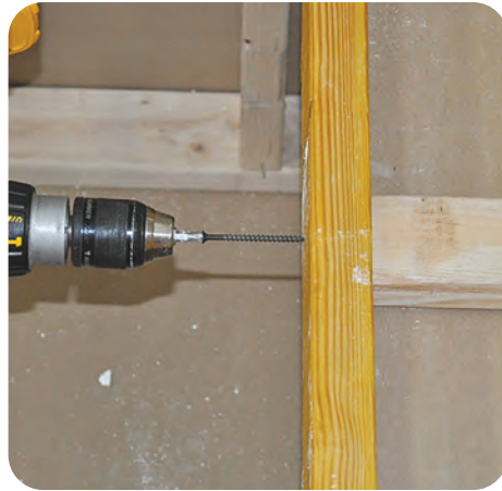
A-2. Attach bracing across joists securely, spacing no more than 24 inches apart
