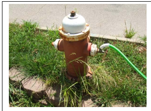
Figure 2-2. Hydrant With Un-metered and Possibly Unauthorized Use.
