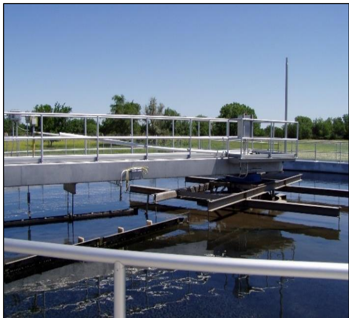
This photo shows a Wastewater Treatment Facility for Lincoln.
