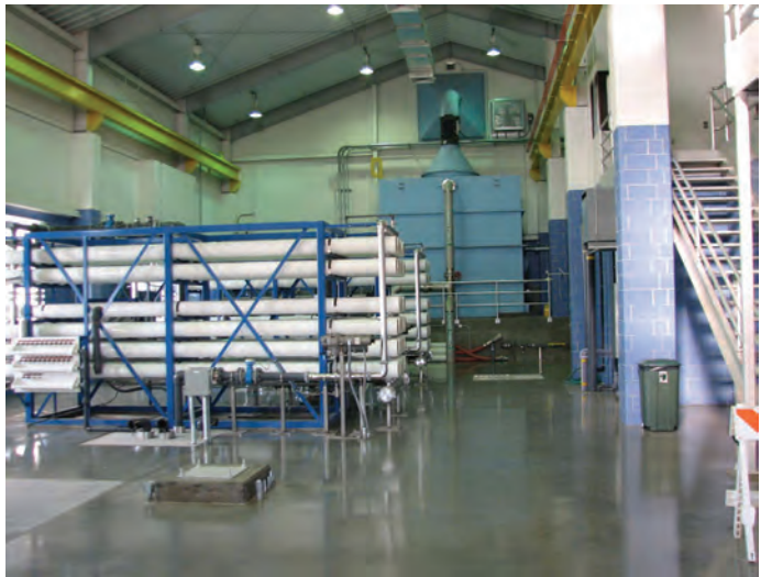
Reverse Osmosis treatment plant to remove nitrate (Seward, NE).
