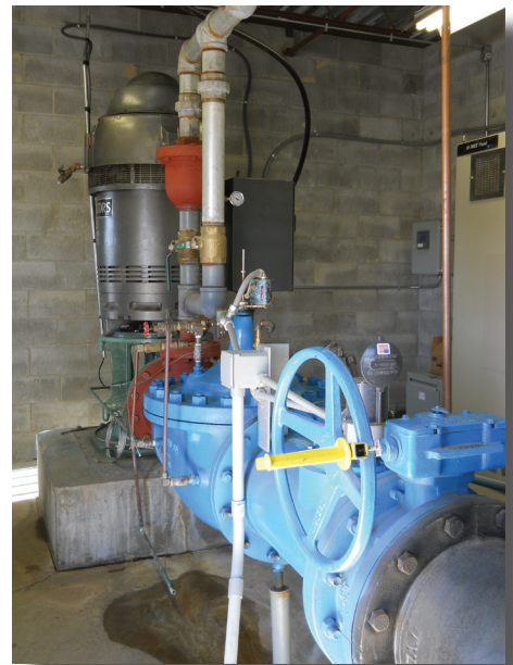
Public Water Supply well capable of pumping thousands of gallons per minute (Hastings, NE).
