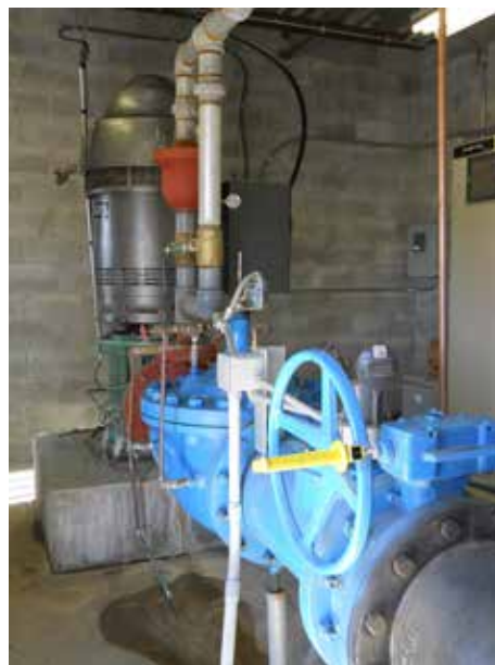
Public Water Supply well capable of pumping thousands of gallons per minute (Hastings, NE).
