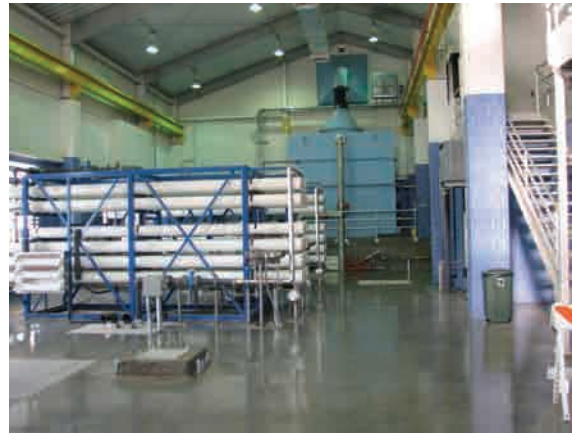
Reverse Osmosis plant to remove nitrates (Seward, NE).
