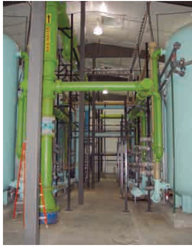
Ion Exchange plant to remove nitrates (McCook, NE).
