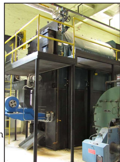
Wood boiler installed at Nebraska College of Technical Agriculture in Curtis, NE
