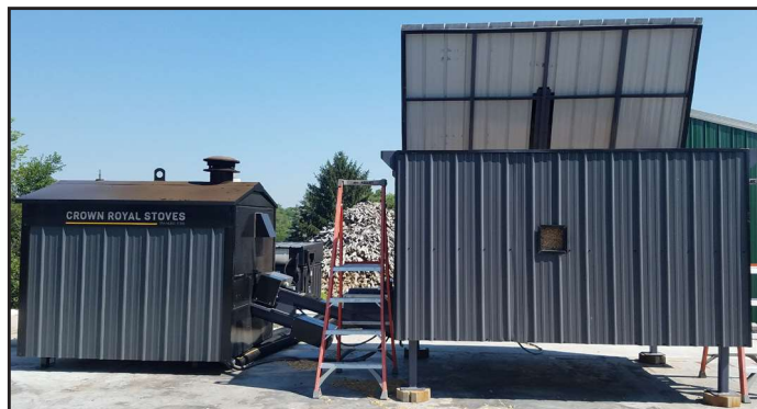
Small woodchip heating system used to provide heat for lumber kilns and product showroom at Big Red Sawmill and Firewood in Palmyra, NE
