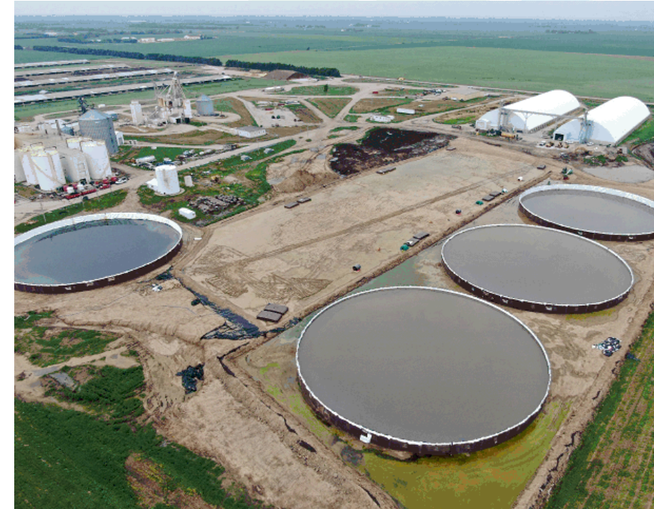
Temporary wastewater storage tanks installed June 28, 2021, LJS
